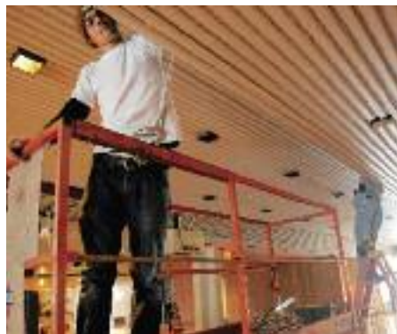
IBEW Local 601 members Stuart Weiss (left) and Chris Lueth (obscured from view) work on a green lighting project at the University of Illinois.
